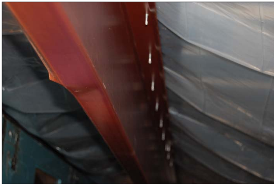
Figure 5.1. Typical Purlin Failure
